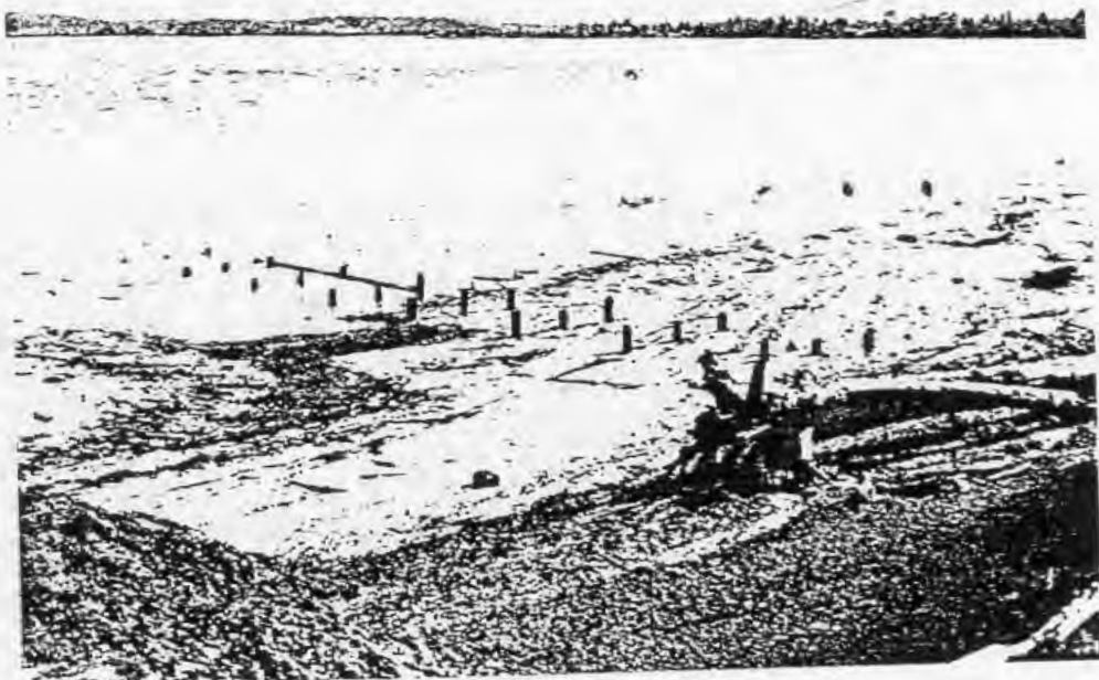
B14-9 Pilings viewed from top of the slag pile. View to the SE. 10BR539
