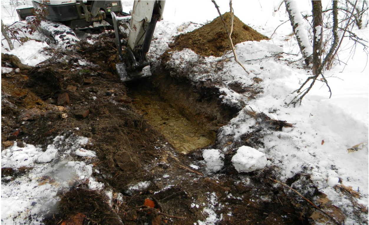
Figure 7. Photograph of TP2 taken during the initial stages of excavation. The I-beam is in the lower center foreground to the right of the red brick. The view is to the southeast.
