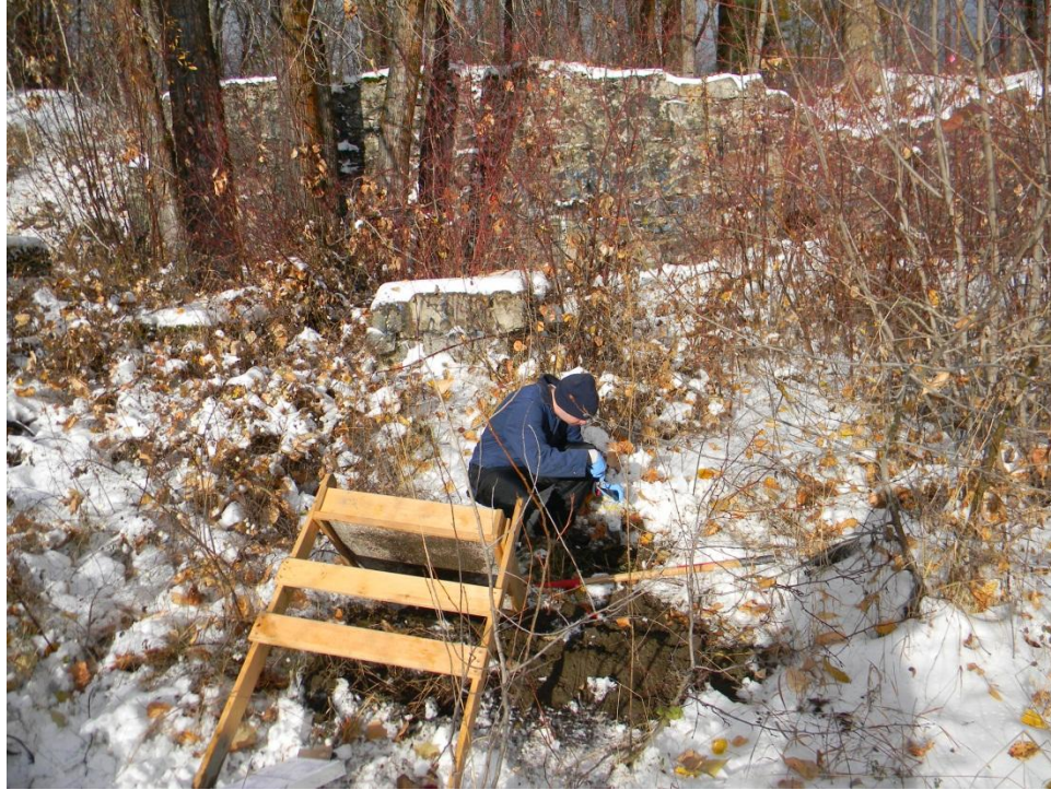
Figure 5. Photograph showing the location of Unit 1 (Z4-FU01-PS01, in the foreground) during excavation. Note the limestone smelter wall in the background. The view is to the northwest.
