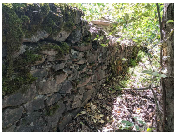
4.) CAREFULLY REMOVE VEGETATION GROWING ON AND AROUND ROCK WALL. EXCAVATE SOIL ON THE NW SIDE OF THE WALL UNTIL 42" OF THE LOWEST POINT ON THE WALL IS EXPOSED. SEE SHEET C8-B FOR GRADING PLAN. SEE SHEET D7 FOR TRAIL AND FRENCH MATTRESS DETAILS.
