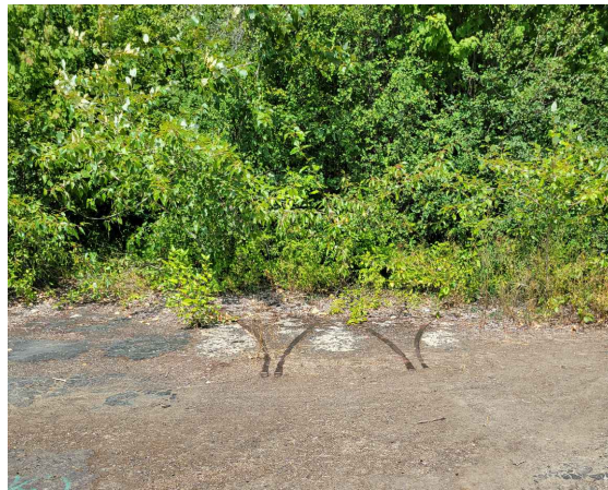
2.) PRESERVE AND PROTECT. CLEAN OUT AND EXCAVATE SOIL AROUND THE EXISTING SLAB AND METAL RAIL IN PREPARATION FOR NEW BLACK ROCK CONC SLAB. FORM CONCRETE AROUND EX. SLAB AND RAILROAD TRACKS. SEE SHEET C3-A
