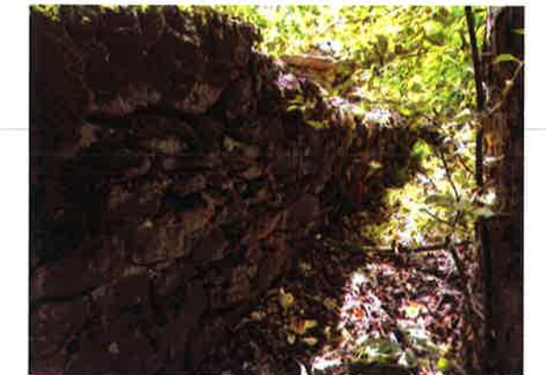
4.) CAREFULLY REMOVE VEGETATION GROWING ON AND AROUND ROCK WALL. EXCAVATE SOIL ON THE NW SIDE OF THE WALL UNTIL 42" OF THE LOWEST POINT ON THE WALL IS EXPOSED. SEE SHEET C8-B FOR GRADING PLAN. SEE SHEET C6 FOR TRAIL AND FRENCH MATTRESS DETAILS.
