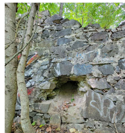
3.) REPAIR EXISTING HOLE IN 2' WIDE ROCK WALL. REMOVE LOOSE MATERIAL AND DIRT BEFORE REPAIRING. USE EXISTING ROCKS IN SITE AREA TO REPAIR WALL. USE TYPE "N" MORTAR.
