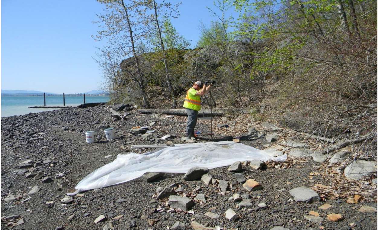
Figure 10. Photograph of SS-4 during excavation. Note Black Rock in the center background and the dock in the left background. The view is to the west.
