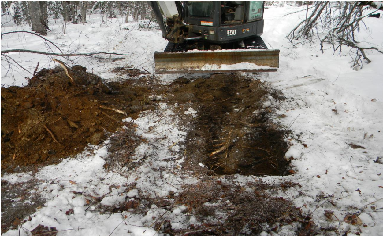
Figure 9. Photograph of TP 3 taken at the start of excavation. The view is to the north.
