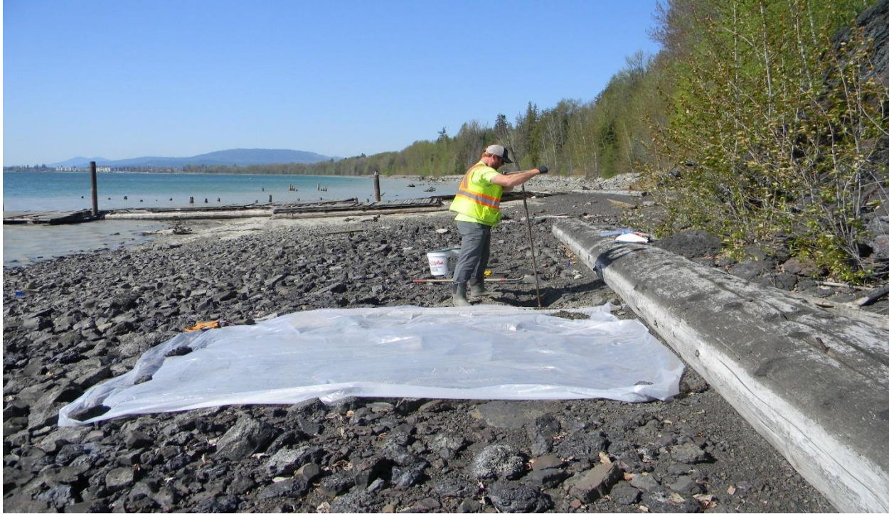
Figure. 6 Photograph of SS-2 during excavation. Note Black Rock at the right and the dock in the left background. The view is to the west.
